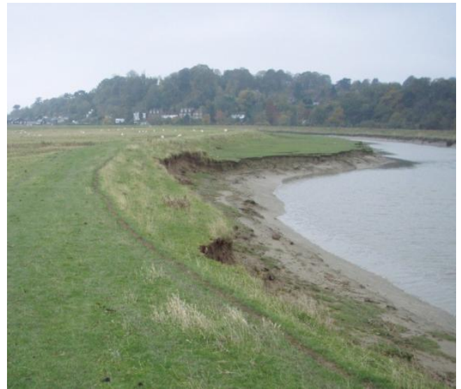
Flood bank erosion on the tidal River Rother
